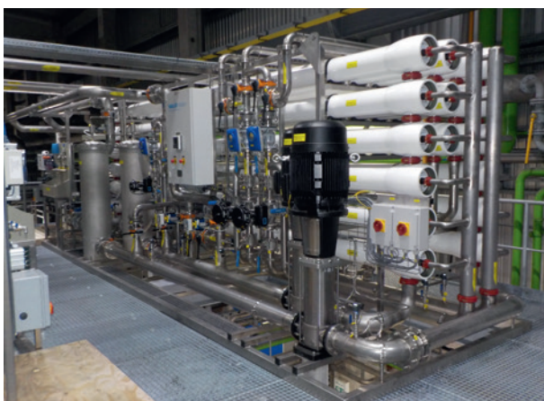
New water treatment plant with reverse osmosis modules
